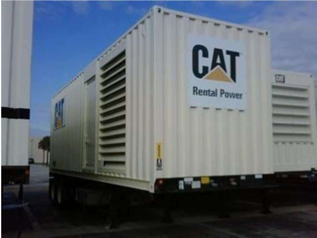
CAT DIESEL GENERATOR
