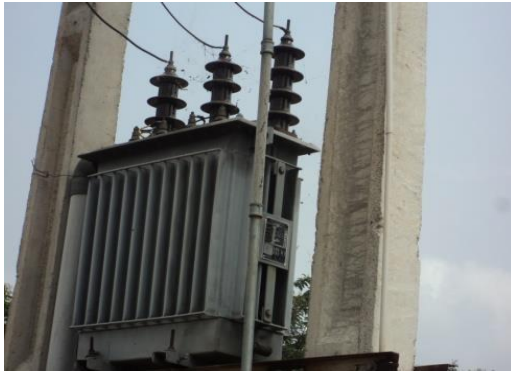
Pole Mounted 100KVA transformer
